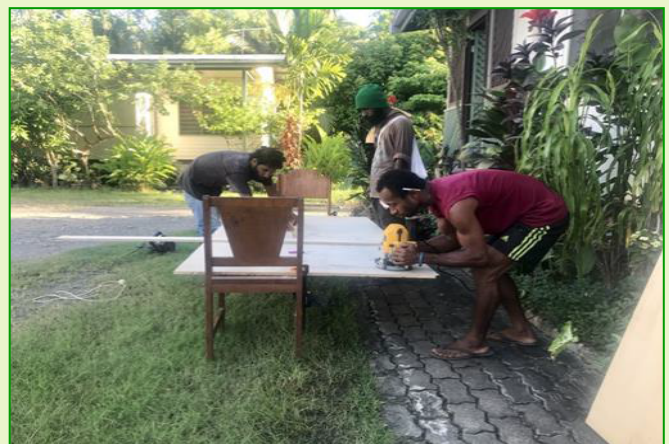
Below; Work being done on the wardrobes and the house by Ignatius and his team.
